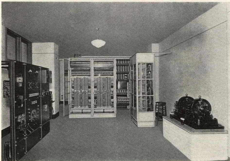
A Typical Type 7 P-A-X Installed, Capacity 300 Lines
