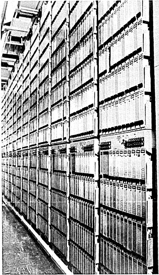
Fig. 27—REG bays, South Knoxville, Tennessee, central office.
